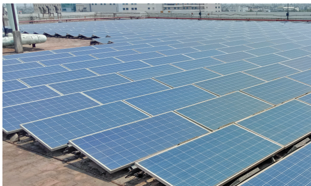
Roof-top solar panels at ICICI Bank Towers in Ambattur, Chennai.
