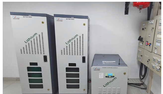
A lithium ion battery storage system at an ICICI Bank branch in Delhi.
